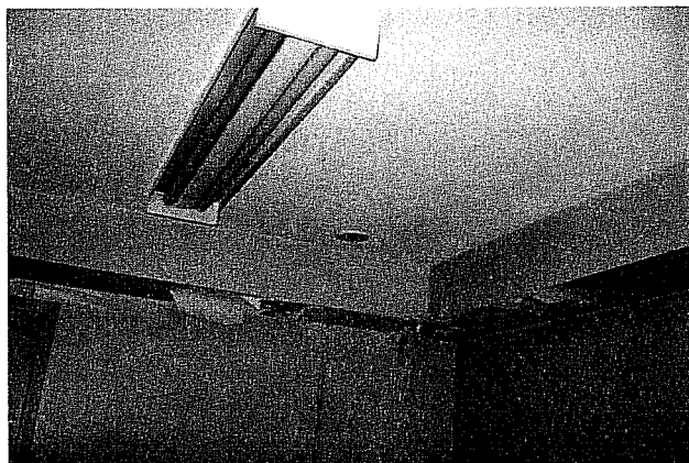
5. View of water damage in 3 rd floor meeting room kitchen.
