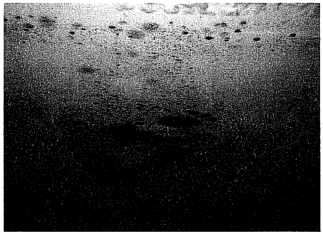
8. View of mould on ceiling of 2 nd floor parking garage.
